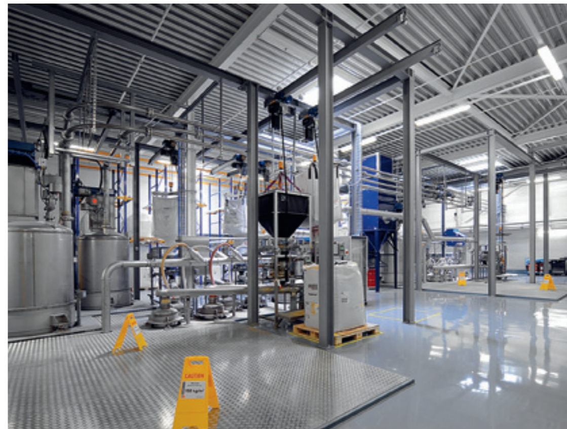
RECOVERING WASTE HEAT, SIKA MANUFACTURING PLANT DUEINGEN, SWITZERLAND
