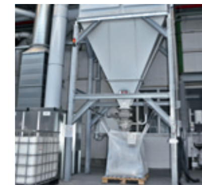
REUSE OF FILTER DUST IN PRODUCTION, SIKA GERMANY PLANT ROSENDAHL, GERMANY
