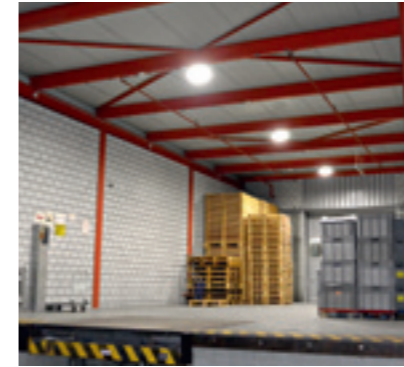
FACTORY AND WAREHOUSE RELAMPING, SIKA EMEA MULTIPLE SITES ACROSS EUROPE
